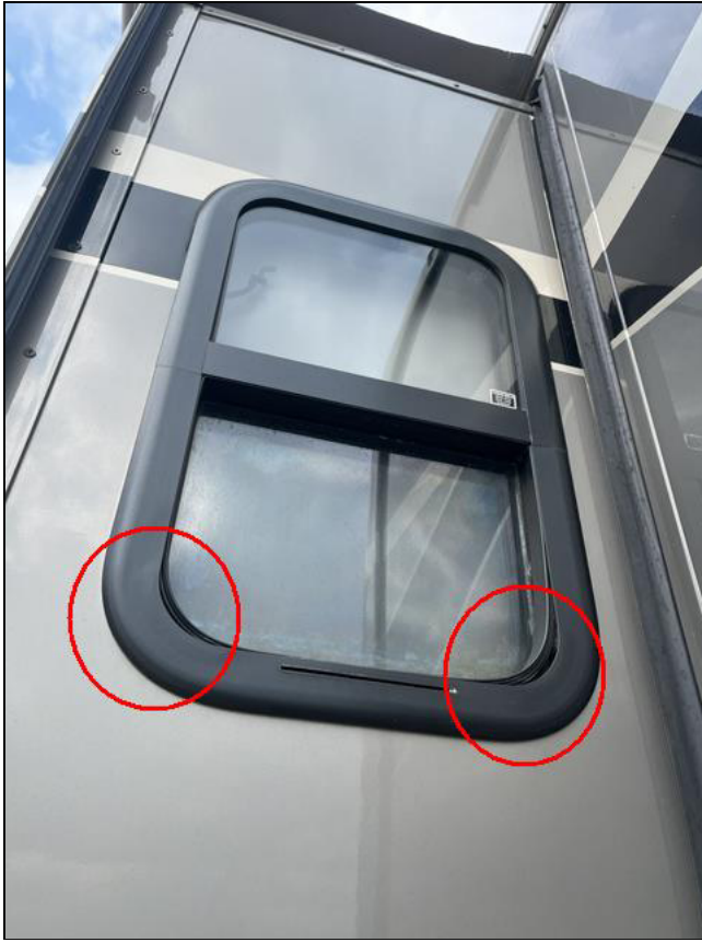
Decaying window seals
