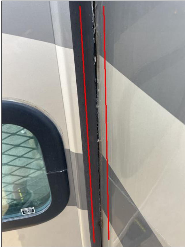
Deteriorating Sealant near door
