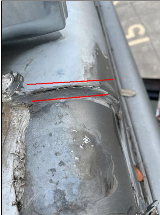
Crack in cap
