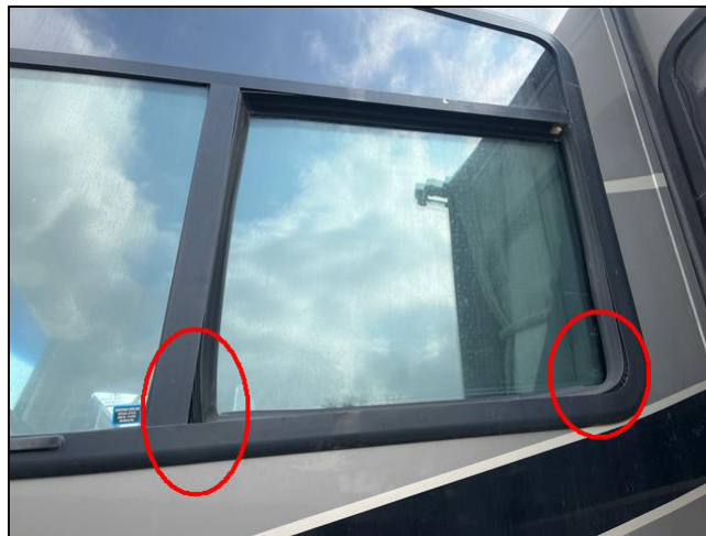
Decaying window seals
